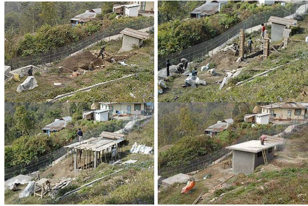
Karmapa orders to buildup a small house for the generator - meanwhile the generator is installed inside and supplies both buildings of the university.
